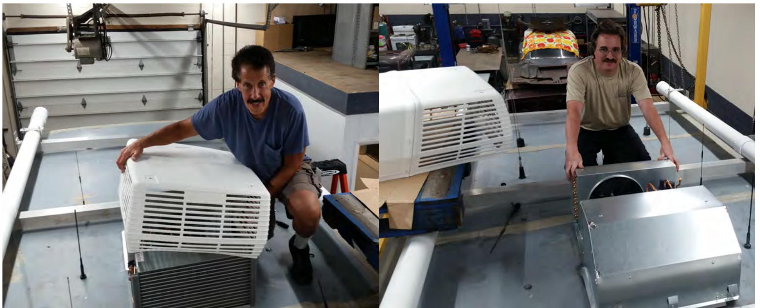
Bob, W2YW and John, W2HCB on the trailer roof with the unit, prepare to make the opening and fit the unit in place
